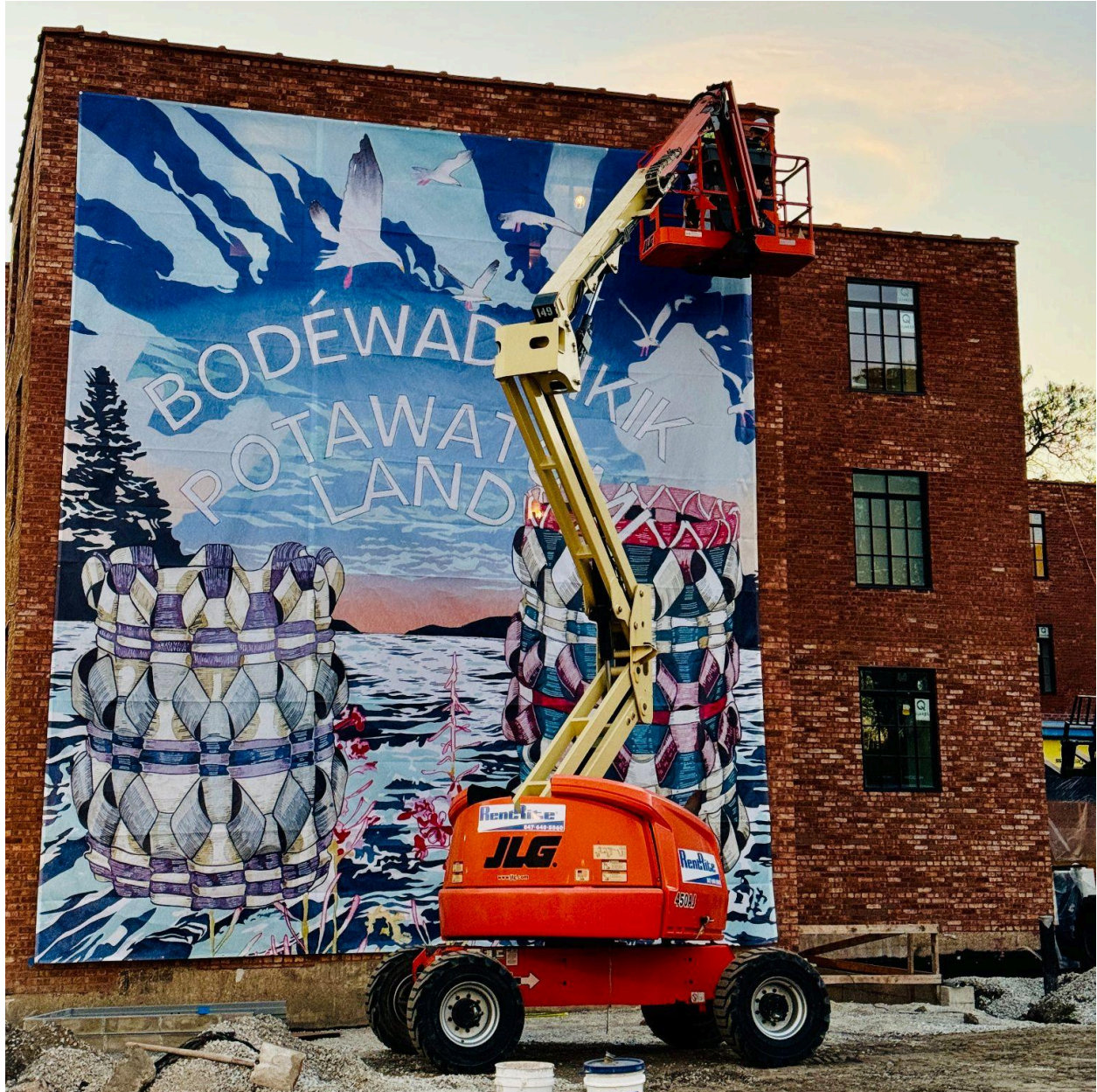
Installation of Invitation Wall mural Still Here: Zhegagoynak by Andrea Carlson. Photo courtesy of The National Public Housing Museum.
